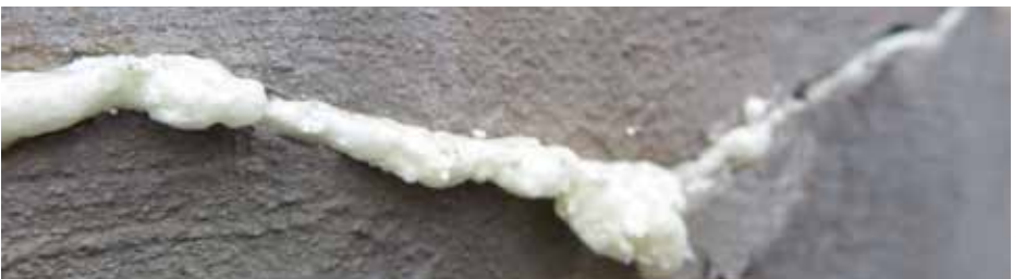
Figure 34. Foam wall crack
