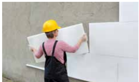
Figure 25. Wall foam insulation to save heating energy
